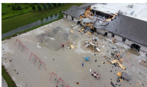
Wind damage at Bishop Baraga School in Michigan. Source: NWS Gaylord/ Jim Chimner
