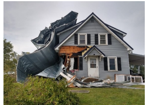
Storm damage near Vinton, Iowa Source: NWS/Darrell Werning
