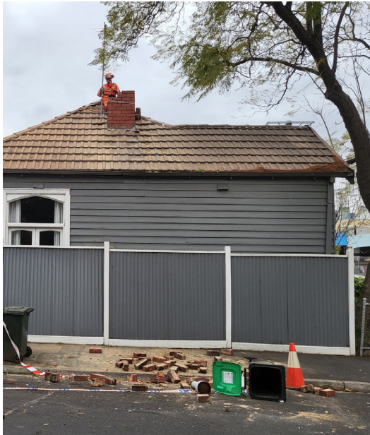
Shingle damage in Essendon, Victoria
