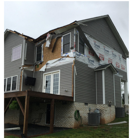
Damage near Wentworth, NC
