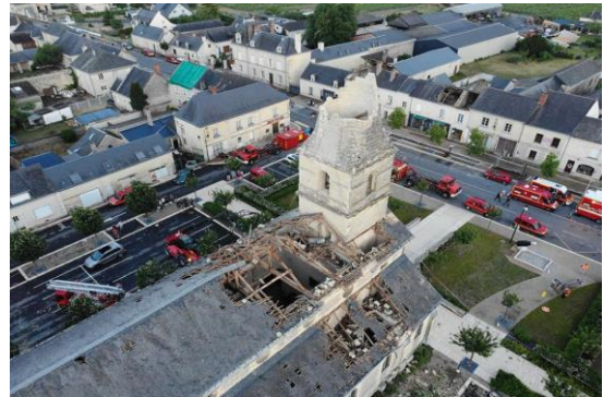
Tornado damage in Saint-Nicolas-de-Bourgueil Source: Indre-et-Loire Fire and Rescue
