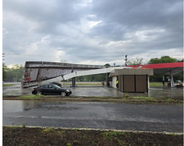
Straight-line wind damage in Rock Hill, SC
