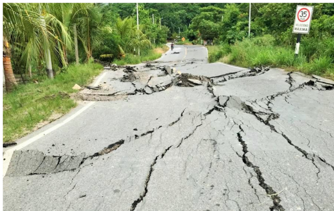
Damage to Peru's Paita-Yurimaguas highway
