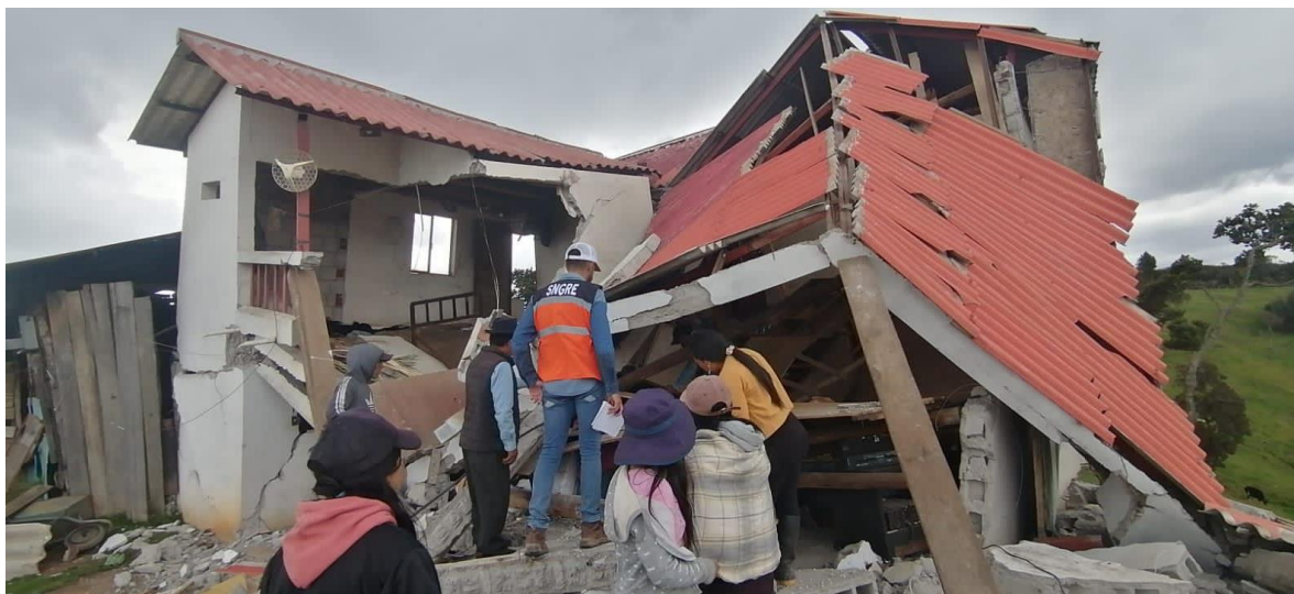
Earthquake damage in Cuenca, Azuay Province
