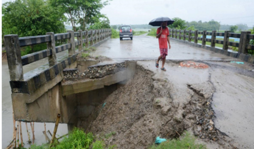
Damaged bridge in Nalbari district of Assam (Source: Press Trust of India)
