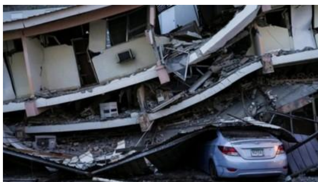
Collapsed building in Penonomé.
