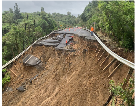
Infrastructural damage near Coromandel Town
