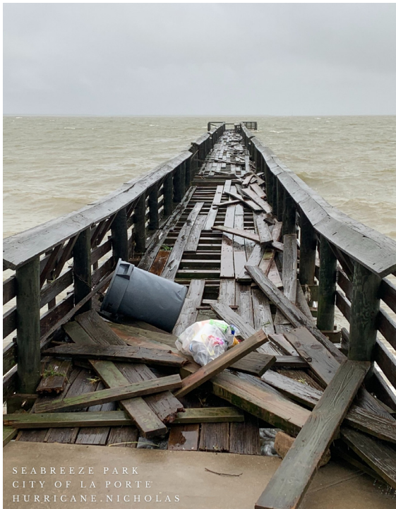
Pier damage at La Porte, Texas
